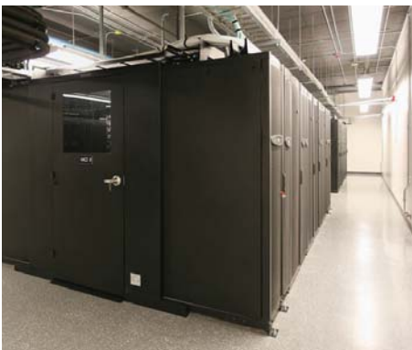
Large IDC/EDC equipment rooms
